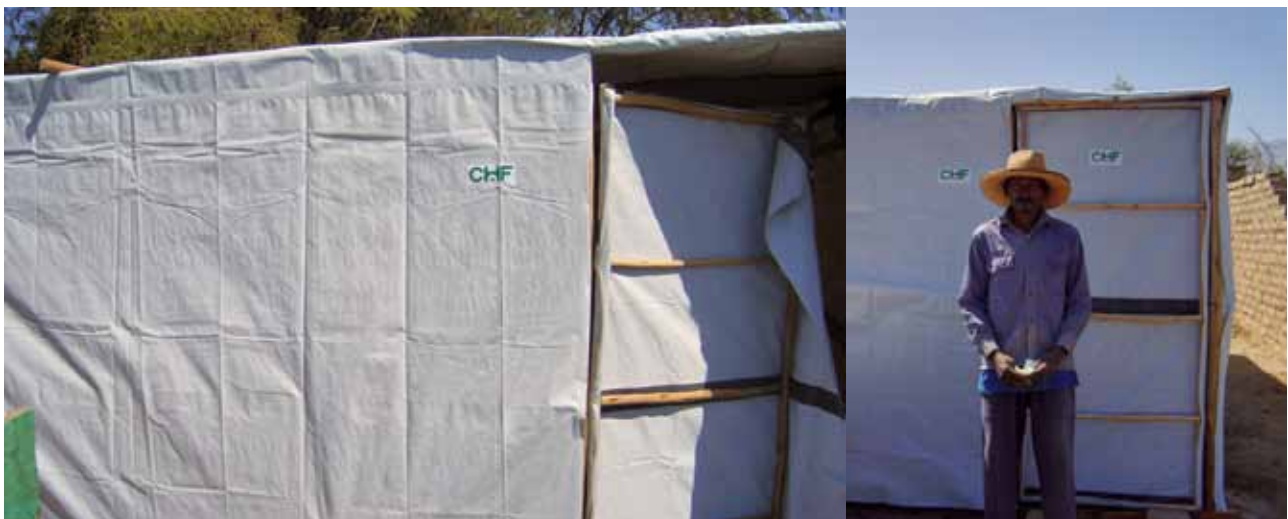
The organisation provided materials and some carpenters to help with the construction. Photos: Eddie Argenal
