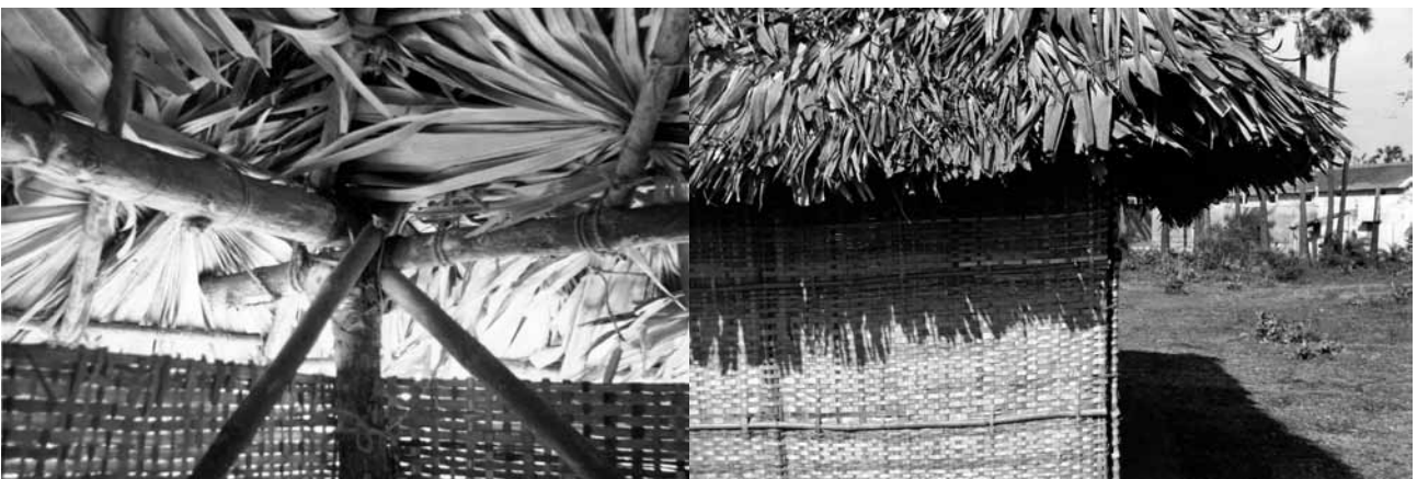
Details of a model home built out of bamboo and thatch to explain a safer techniques in cyclone resistant housing. It had key elements of: a well-anchored central post, triangulation to stiffen the frame, good connections of roof to wall using metal connections Photos: Ian Davis
