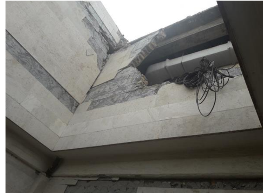
Damage to interior walls, 2017 Kermanshah earthquake Sarpol'e Zahab Hospital (IIEES-2017).
