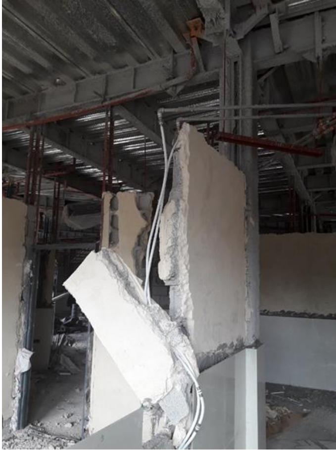
Damage to piping system, 2017 Kermanshah earthquake Sarpol'e Zahab Hospital (IIEES- 2017).
