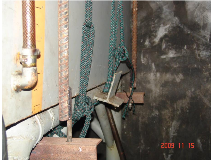
Damage to Diesel Gen. Fuel Tank, 2009 Ache earthquake (2009).
