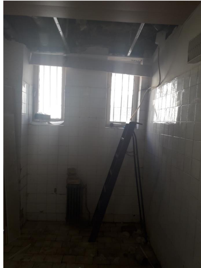
Water pipe breakage, 2017 Kermanshah earthquake Paveh Hospital (IIEES-2017).
