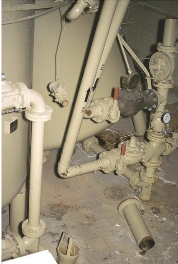
Broken piping in the new powerhouse for the Olive View Hospital, 1971 San Fernando earthquake (NISEE, 2016b).
