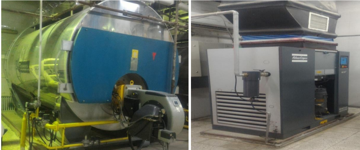
Figure 14 mechanical equipment in Non-Structural assessment
